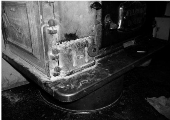
Figure 6: Coal stove in disrepair (b)
